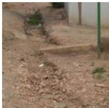
Figure 12: Example of stormwater damage in Otjomuise
