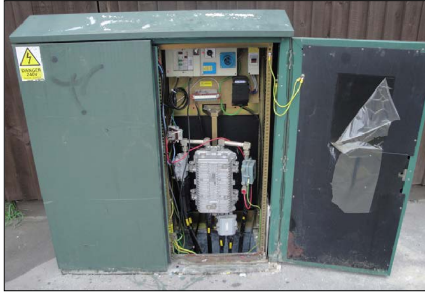
Figure B102 - Feeder Pillar Next to Wiltshire Road Bay
