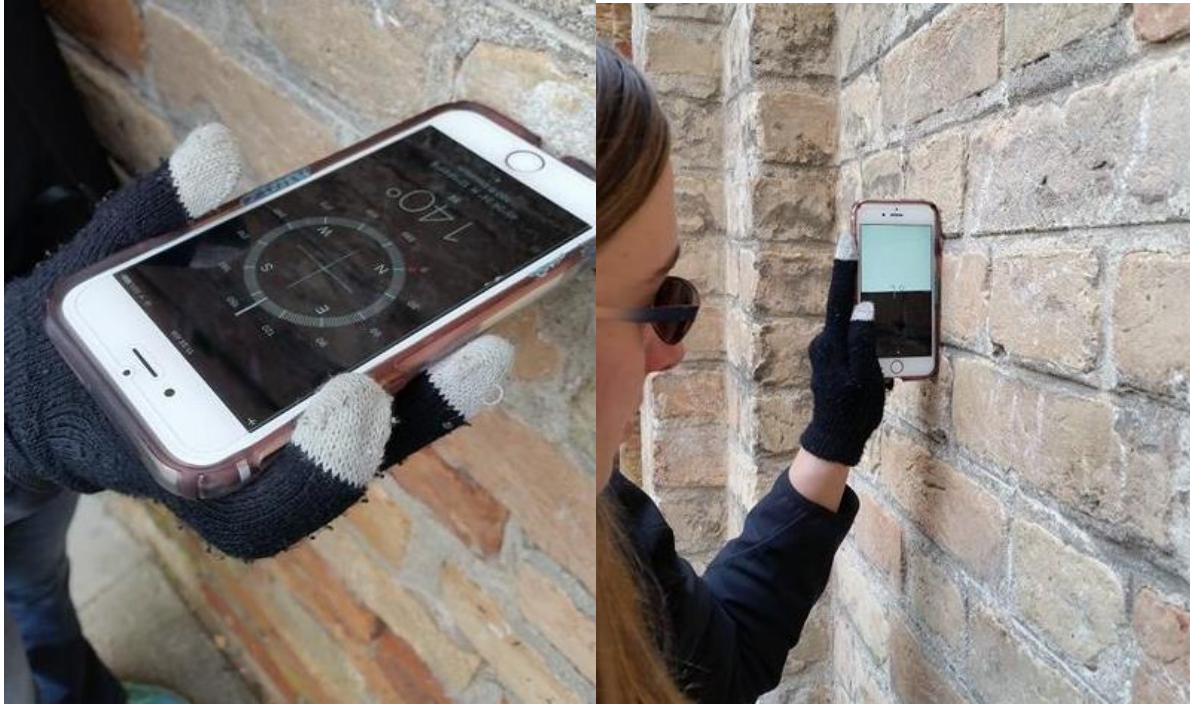
Figure 15 - Left: Measuring the Orientation of the Tower, Right: Measuring the inclination of the a tower
