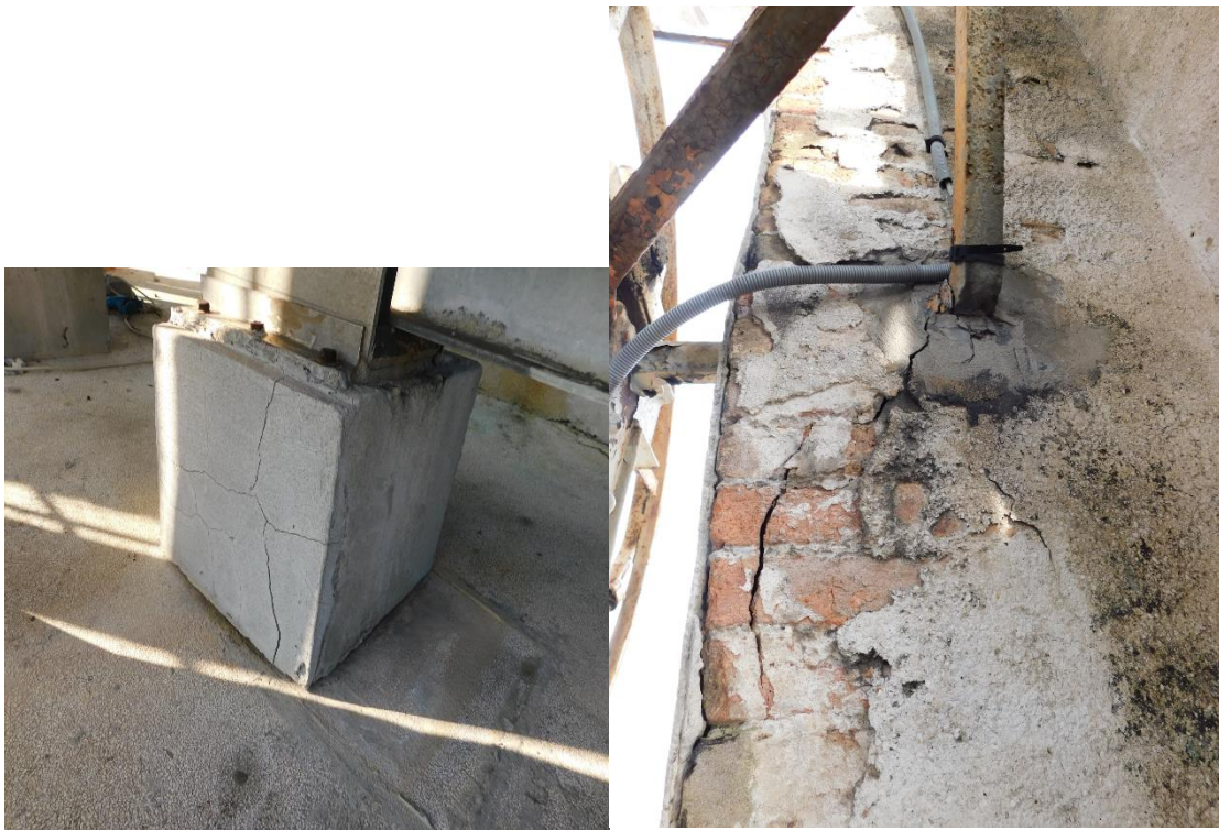
Figure 62 - Cracks from the bell frame in San Giacomo dell’Orio (left) and Gesuati (right)
