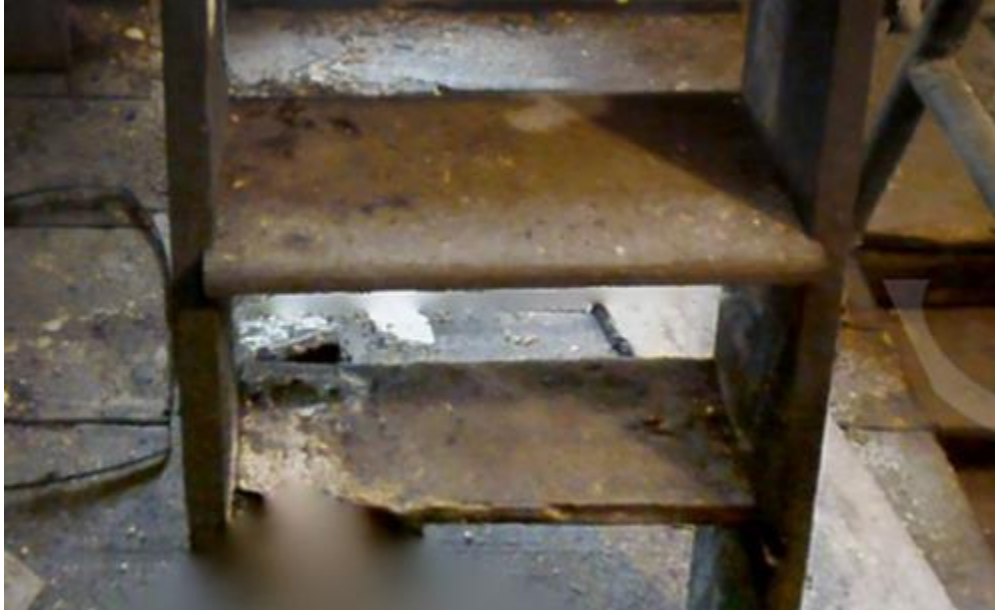
Figure 18 - Example of a bad step in Gesuati
