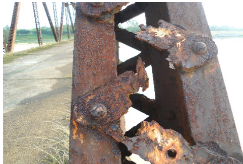
Figure 1: Corrosion on infrastructure. 3
