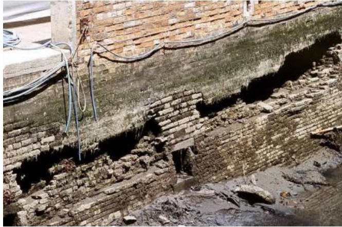
Figure 7: A sboccho, or sewer outlet, revealed in a drained canal for maintenance
