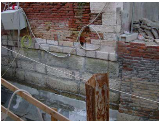
Figure 9: Canal Wall Damage in Venice
