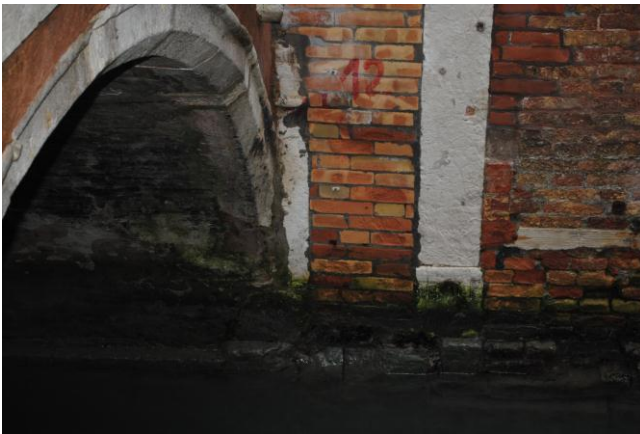
Figure 21: Damage to canal walls
