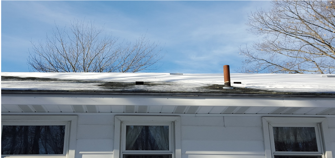
Figure 58: Problematic Small Roof Vents
