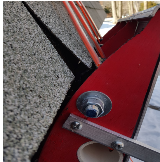
Figure 50: Single Damage with Side-to-Side Movement
