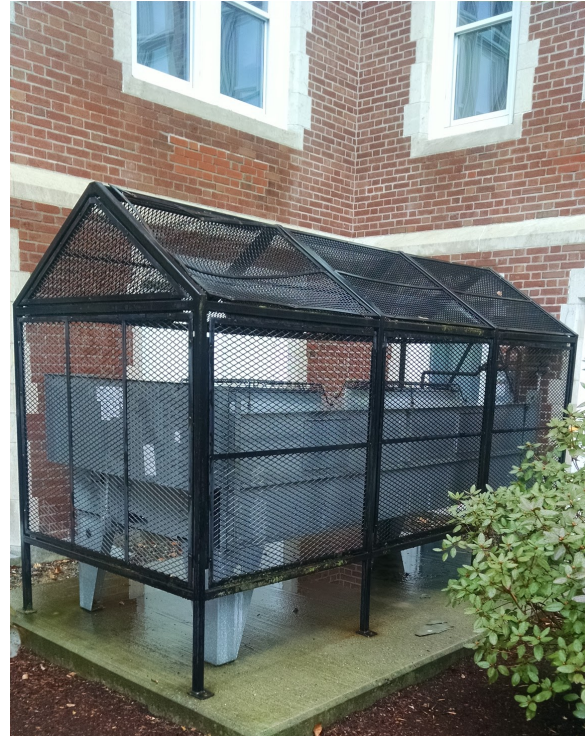
Figure 45: HVAC Grate Used for Testing
