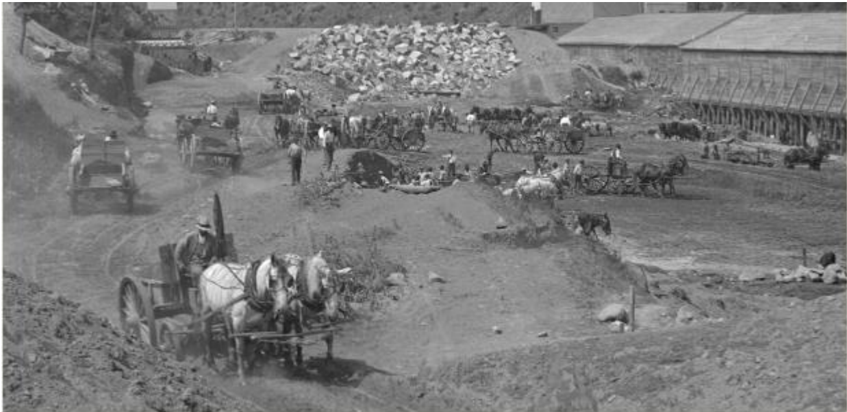
Figure 19: Excavation Techniques from Massachusetts Annual report of the Metropolitan Water Board. c.1 v.6 1900. Retrieved from https://babel.hathitrust.org/cgi/pt?id=chi.72624881&view=1up&seq=9
