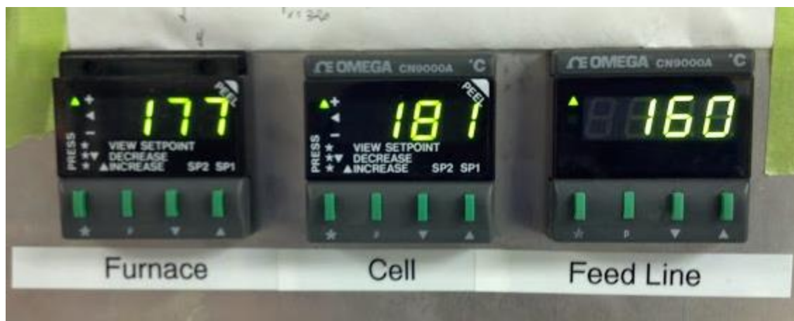
FIGURE 44: TEMPERATURE CONTROL BOXES
