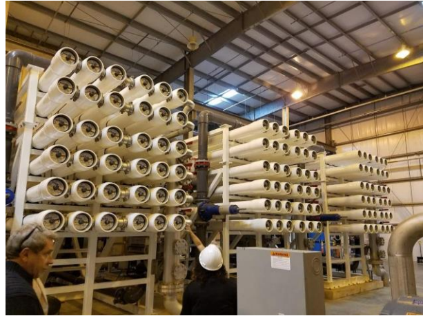
Figure 2: Reverse osmosis trains in TRDF
