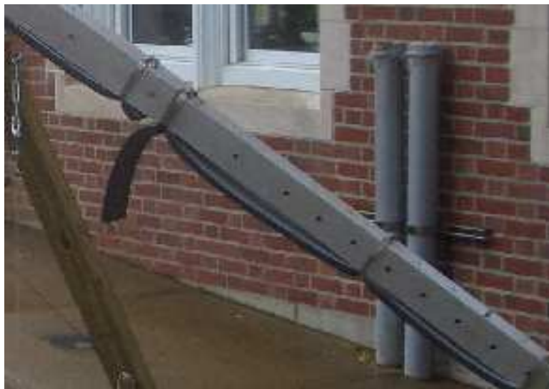
Figure 25: HVAC Duct Lining
