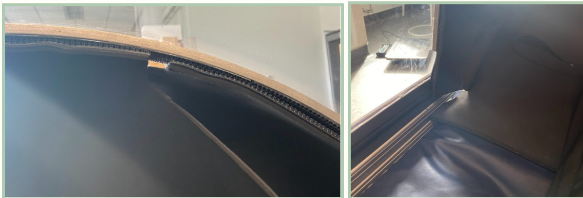
Figures 56 and 57: Sealing Holes at Neoprene Connections on the Top of the Shell and Intersection with Frame, respectively.
