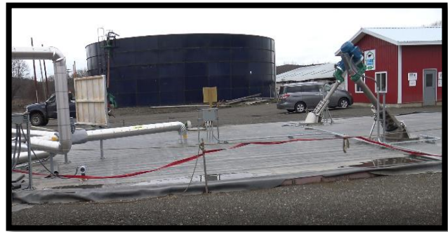
i.) Effluent holding tank with hydrolyzer and mixers in foreground
