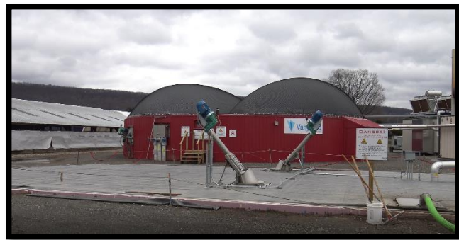
c.) Anaerobic digester with hydrolyzer tank and mixers in foreground
