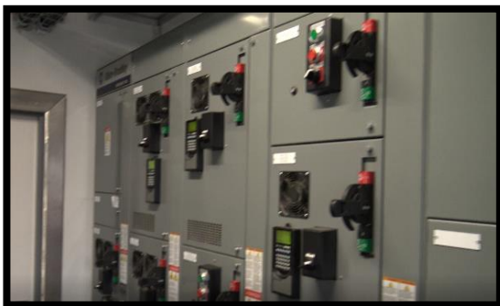
f.) Odor Control Station
