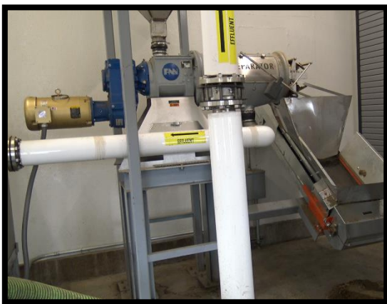
h.) Separator – separates dry digestate and wet effluent
