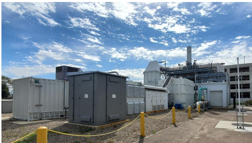
Figure 7: 2.8 MW gas-fed molten carbonate fuel cell at UC San Diego.
