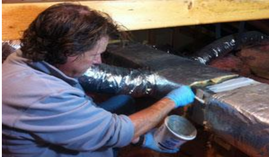
Figure 8: A typical air duct sealing procedure. http://www.goodmanphc.com/ . (Goodman Plumbing, Heating & Cooling, 2015).
