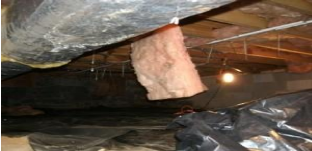
Figure 11: A crawlspace that needs some attention or treatment (before weatherization). http://edge-gogreen.com/home-performance/home-performance-and-weatherization/crawlspace-weatherization/ . (EDGE Energy, 2015).
