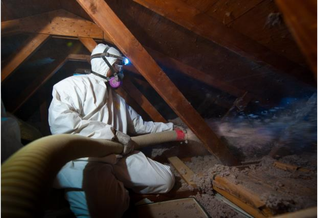
Figure 6: An insulation professional filling the attic of a home with blown-in insulation. A respirator is used because certain types of insulation can be hazardous to the lungs and so one must adhere to all manufacture safety warnings. http://www.greenbuildingadvisor.com (Green Building Advisor, 2015).
