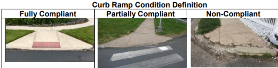
Figure 9: Provides photos to demonstrate what sidewalks and curb ramps could look like with the corresponding categorization.
