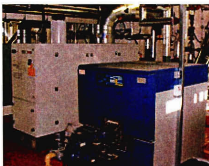
Figure 5: An Installed CHP System
