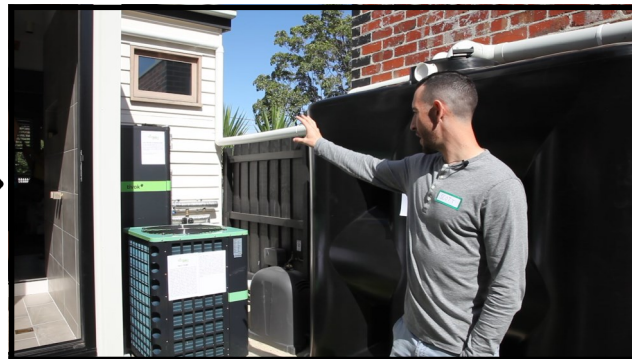
“The engine room of our sustainable home...” “Our Heat Pump and Storage Tank...”
