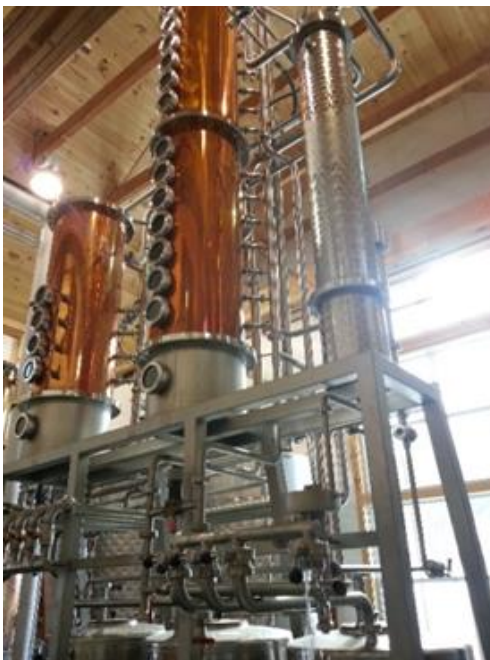
Figure 5: American Crafted Spirits Distillation Columns and Condenser
