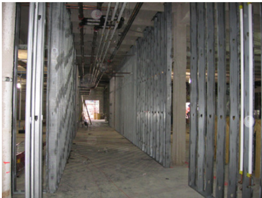
Figure 2.19: Photograph showing the exposed metal studs during a renovation in Atwater Kent Laboratories
