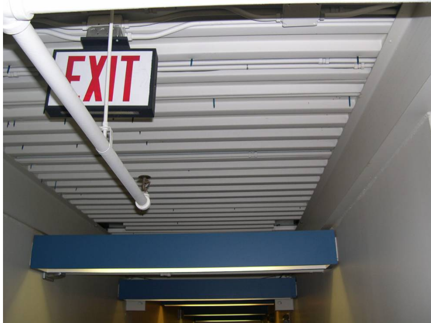
Figure 2.18: Photograph showing the metal ceiling and floor decks in the Atwater Kent building
