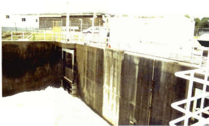
Figure 12: Excessive Turbulent Flow on VY Sluice Gate
