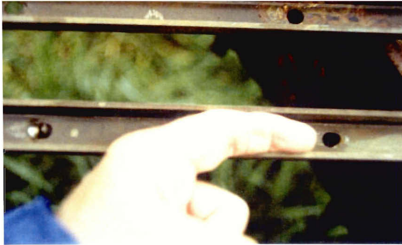
Figure 11: Damaged Tongue Liner
