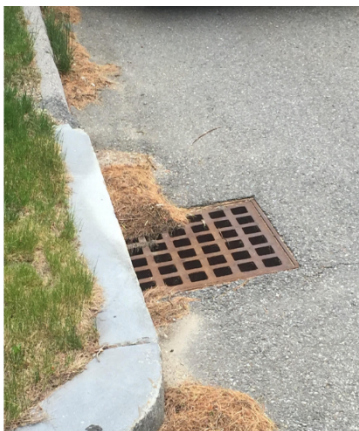
Figure 10: Example of a catch basin in the town of Holden
