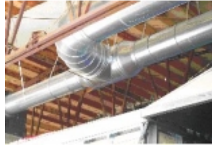
Figure 3-10: Union in Ductwork
