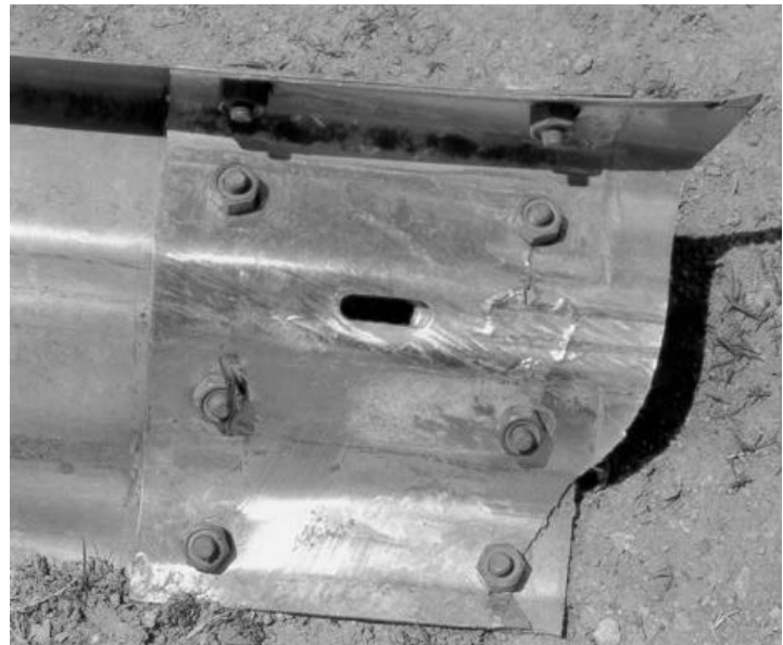
Figure 37: Ruptured rail element in TTI test 405541-4.(18)
