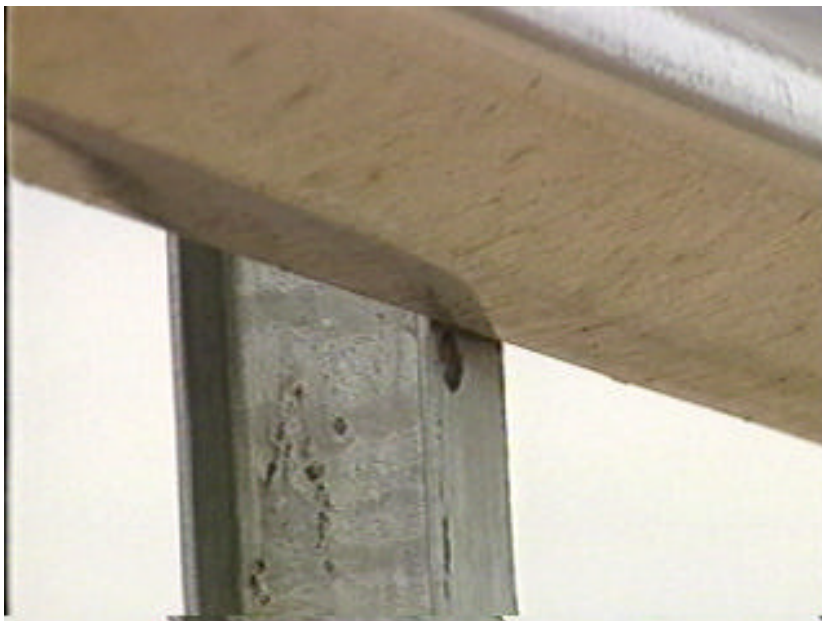
Figure 79: Eliminated shelf bolt.
