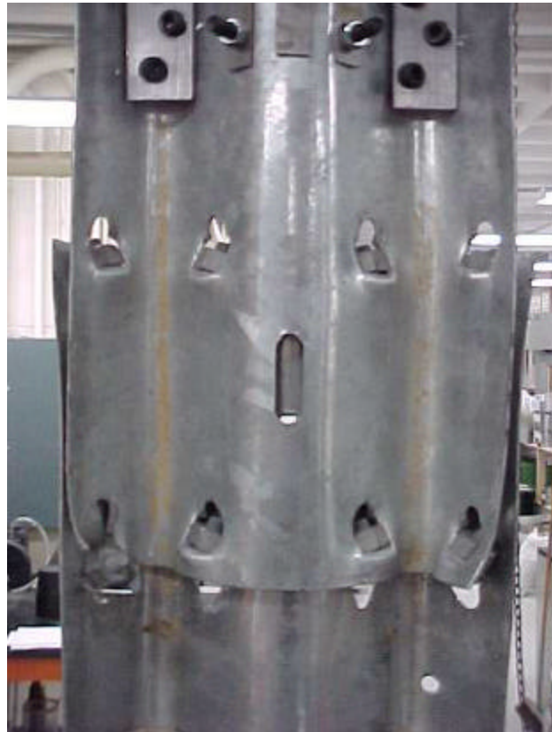
Figure 10: Failed splice connection.
