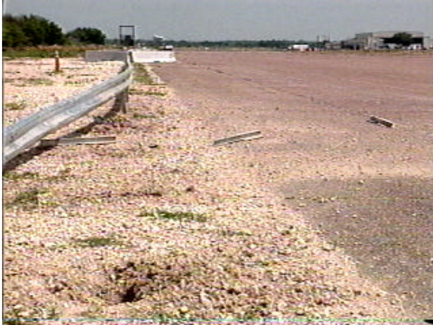
Figure 104: Posts pulled out from the ground.
