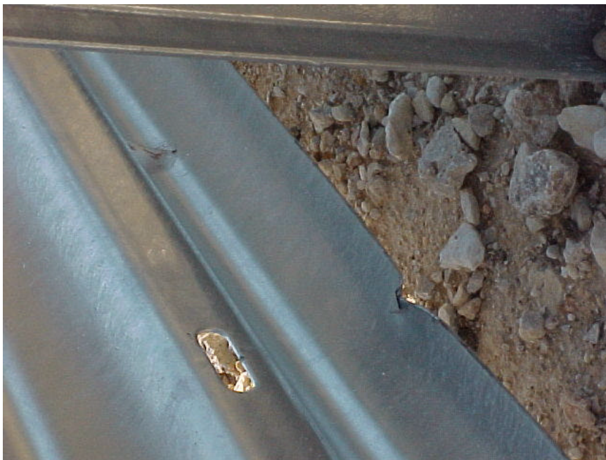
Figure 57: Rail deformation at a post.(9)
