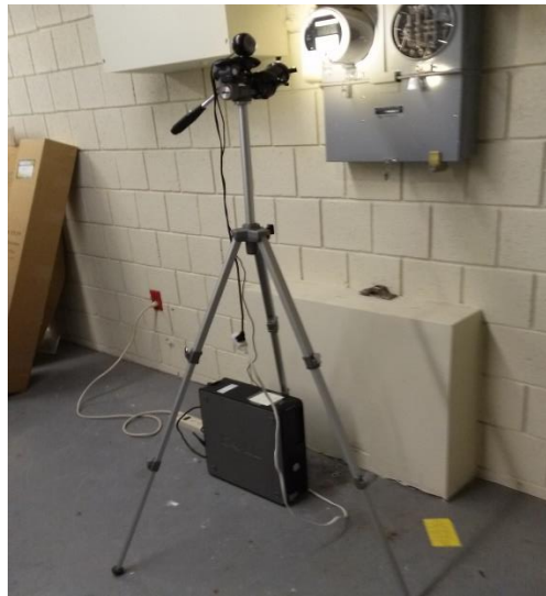
Figure 24: Founders Hall electric metering webcam setup
