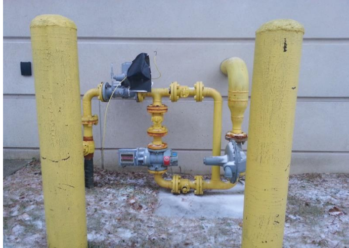
Figure 23: East Hall Gas Meter
