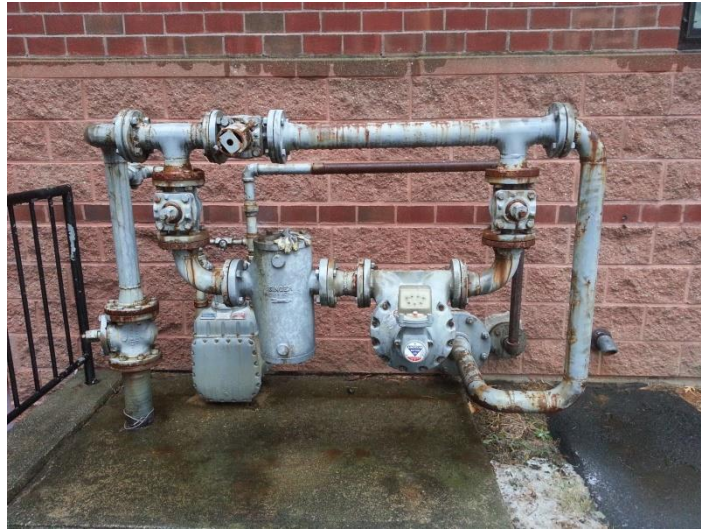
Figure 16: Founders Hall Gas Meters
