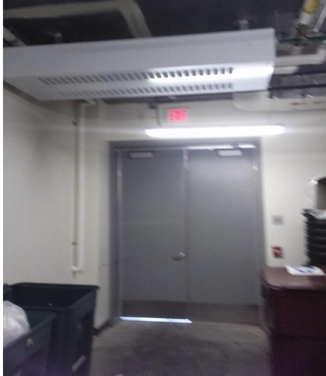
Figure 15: Gap in East Hall Main Trash Room door
