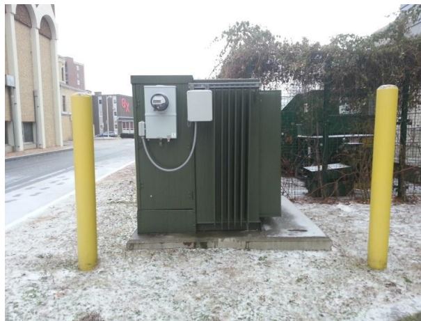
Figure 22: East Hall Electric Meter
