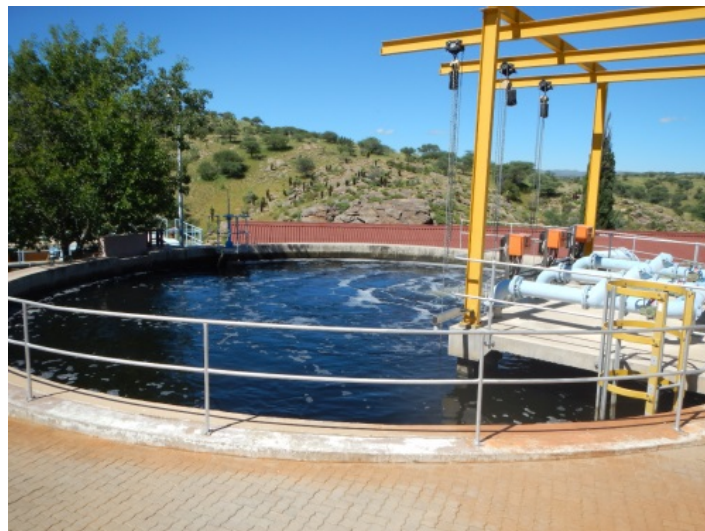
Figure 3: Windhoek's water reclamation plant. Source: Colby Foster (WPI Student), used with his permission.
