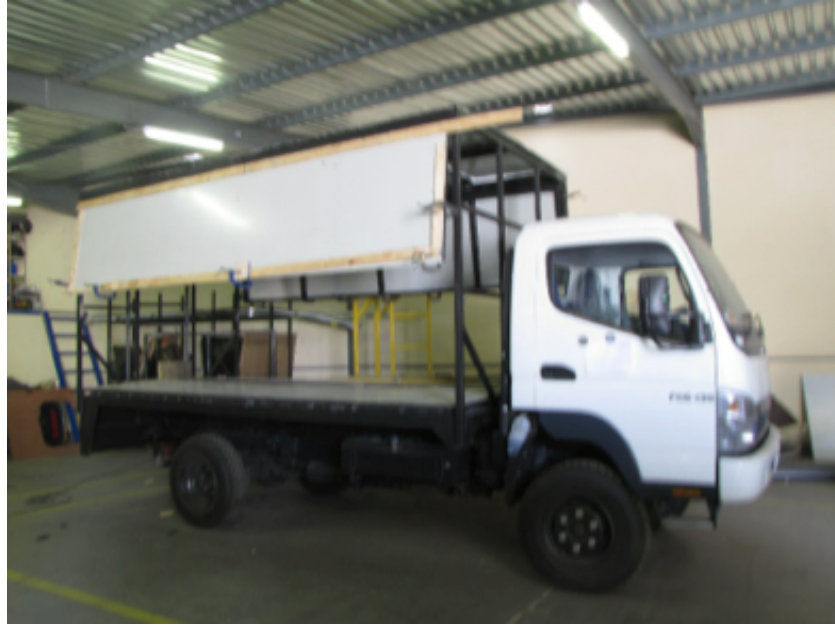
Figure 6: The EduMobile truck under construction. Source: Tauno Iipinge, used with EduVentures' permission.
