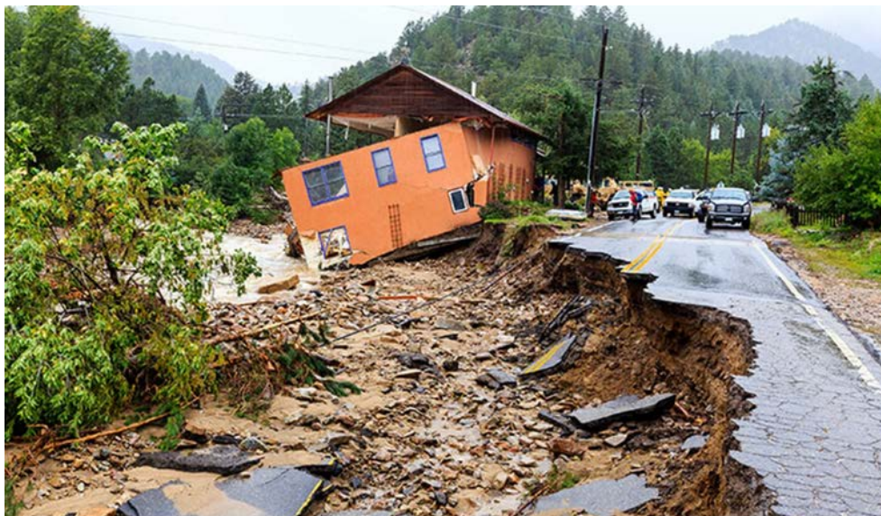
Figure 2.4: Building that collapsed into the stream following the flood in 2013 (Kwak-Hefferan).
