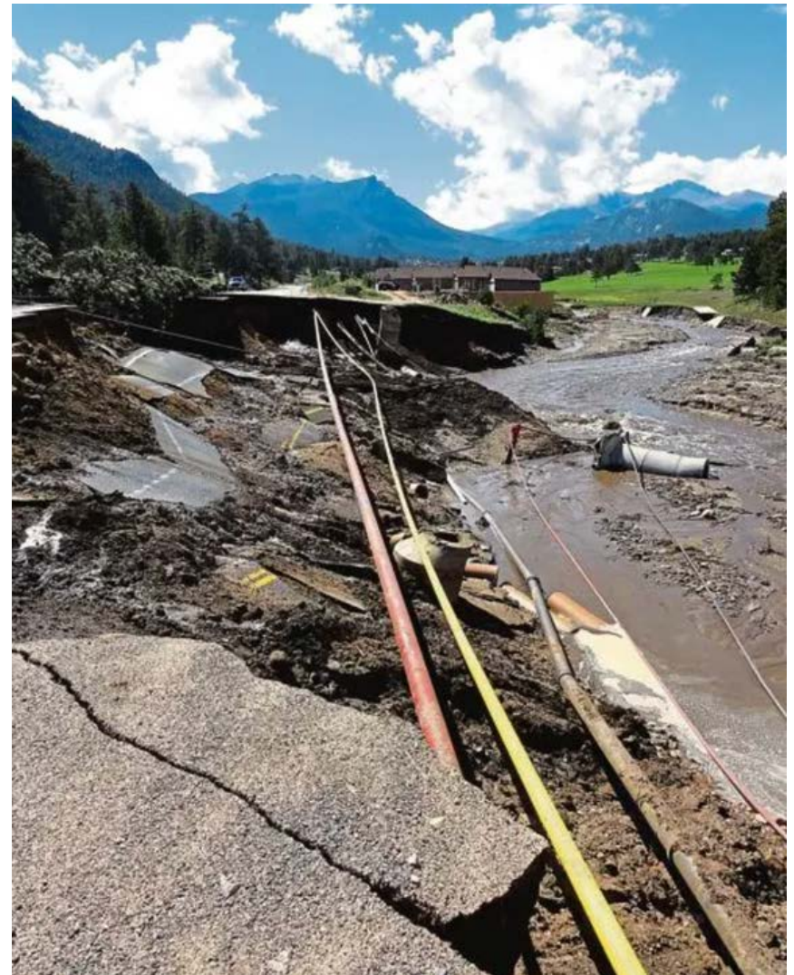
Figure 2.9: Collapsed road after the 2013 flood exposing unearthed pipelines (Town of Estes Park).
