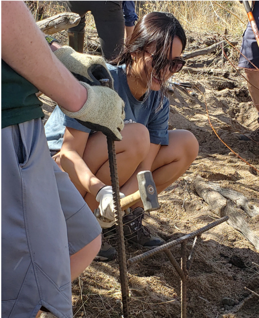
Figure 3.14: Team members staking rebar into the stream banks to prepare for willow planting. Photo taken by Michael Beskid.
