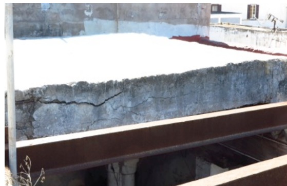
Figure 38: Physical Damage on the roof of Foundouk Al Khayyatene
