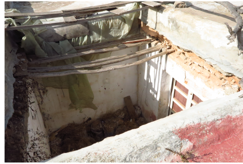
Figure 30 Collapsed room in foundouk Jdilda
