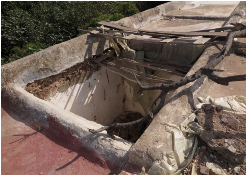
Figure 19 Collapsed Room of foundouk Jilda
