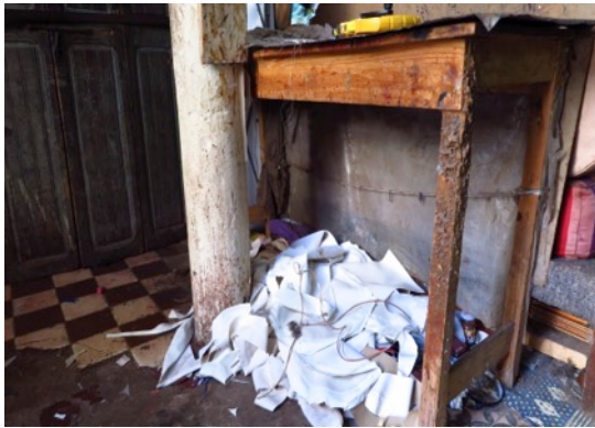
Figure 35 Trash on the floor of Ben Aissa
