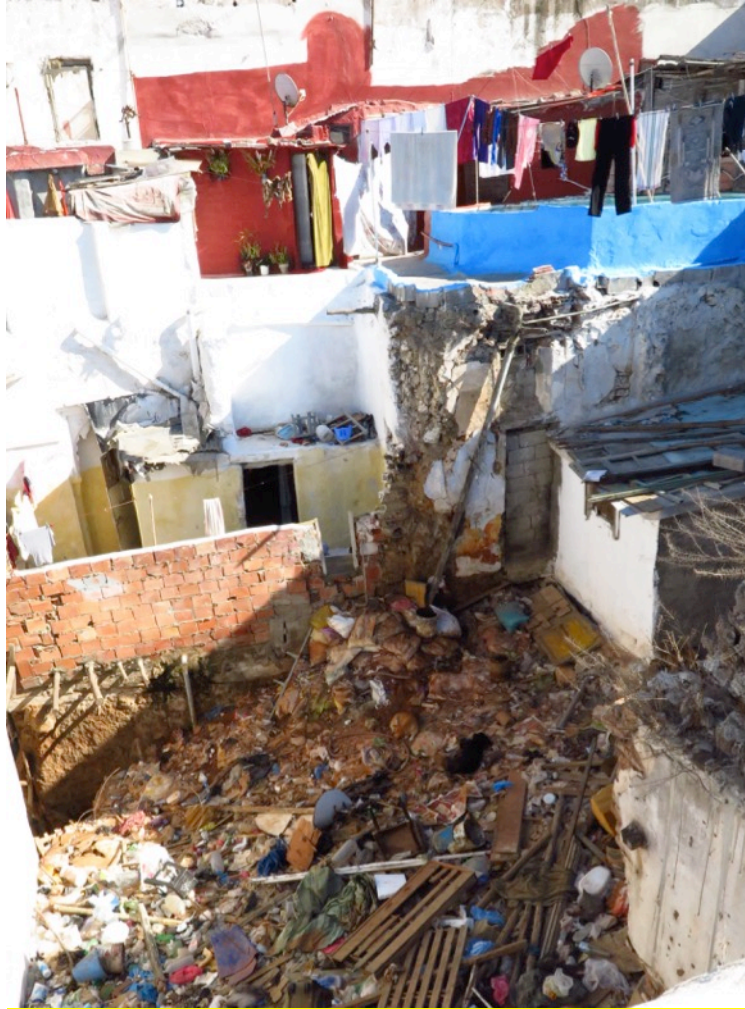
Figure 20. Collapsed Section of Ben Aissa
