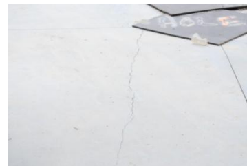
Figure 9: Crack on slab on grade.
