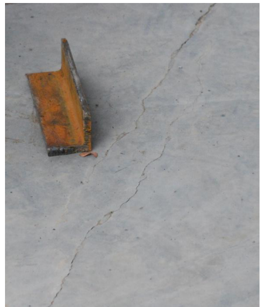
Figure 12: Shrinkage Crack ending and restarting again in parallel on the A Wing slab. Picture taken 11/11/2009.
