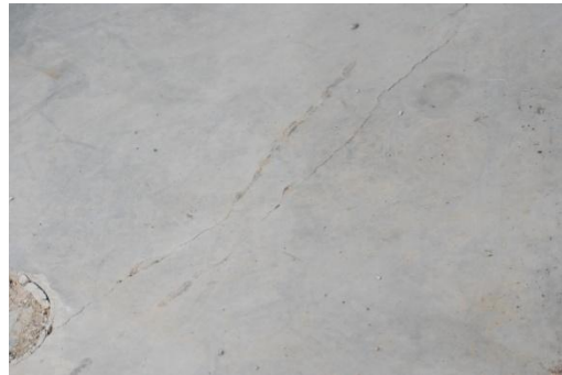
Figure 14: Shrinkage Crack ending and restarting again in parallel on the A Wing slab. Picture taken 11/11/2009.
