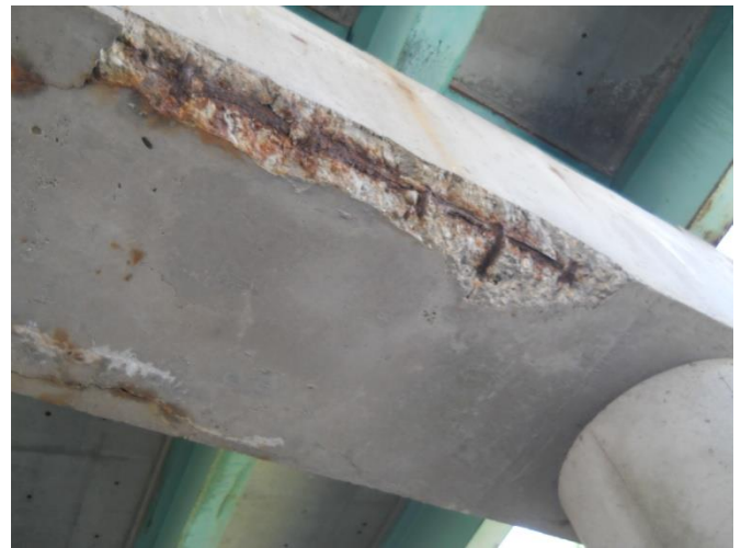
Figure 4: Clear evidence of rust related spalling, reinforcing cage fully exposed in places. This damage is located on the bottom of hammerhead on northern pier of SB Bridge.
