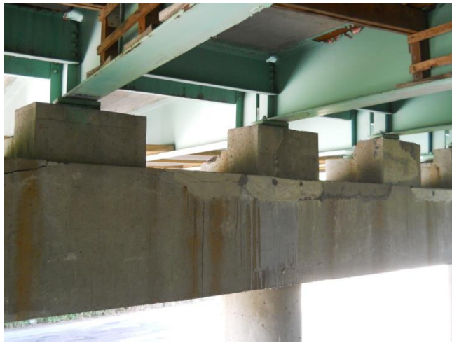
Figure 3: Large number of repaired and current concrete failure locations on the southern pier of the SB Bridge. Note the very evident water staining and continued cracking to the bridge seats.
