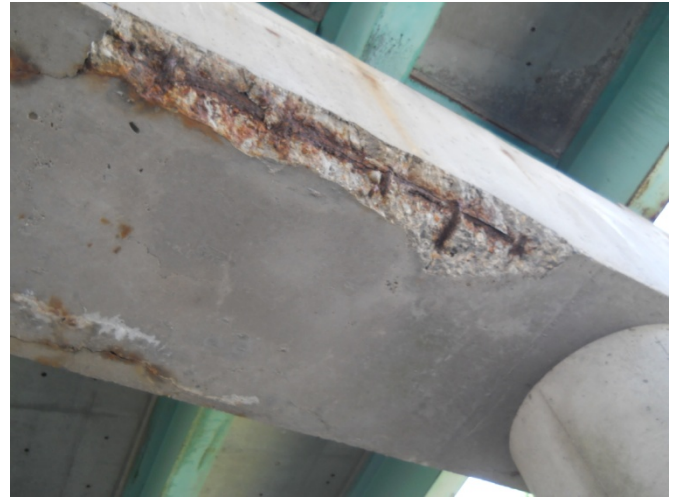
Figure 4: Clear evidence of rust related spalling, reinforcing cage fully exposed in places. This damage is located on the bottom of the hammerhead on the northern pier of the SB bridge.
