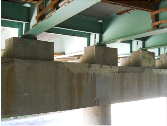
Figure 3: Large number of repaired and current concrete failure locations on the southern pier of the SB Bridge. Note the very evident water staining and continued cracking to the bridge seats.
