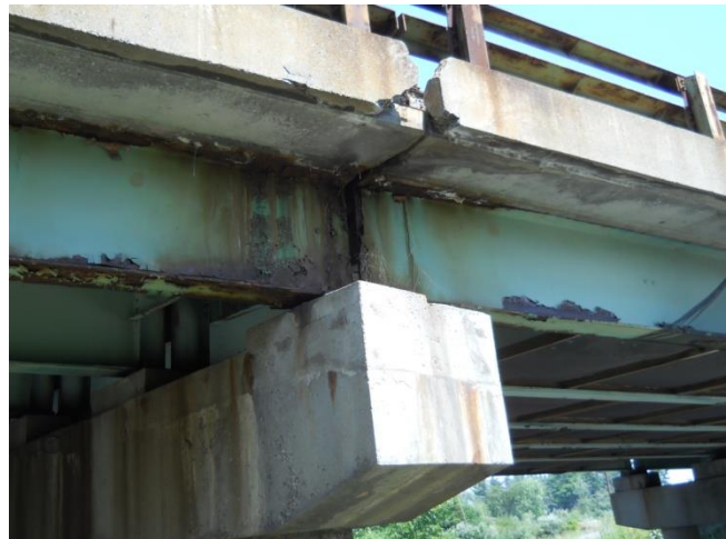
Figure 6: Paint damage and decaying roadway coping. Picture shows the northern expansion joint on the eastern side of NB Bridge.
