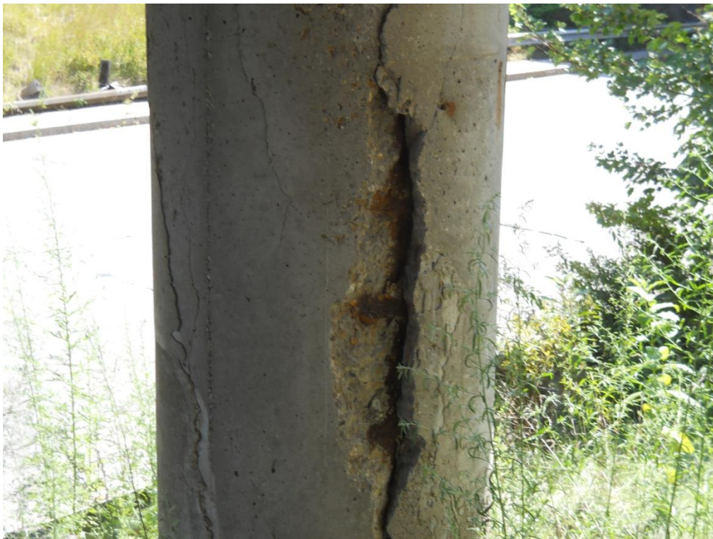
Figure 5: Severe spalling, cracking and separation of concrete cover on a pier on I-93 on the Northbound bridge.
