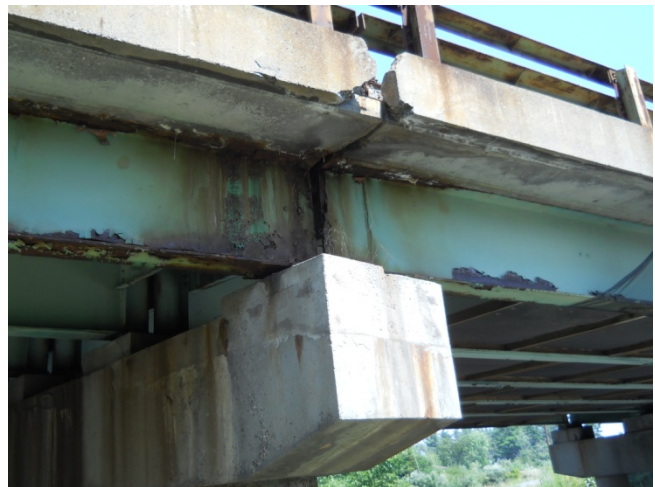
Figure 7: Paint damage and decaying roadway coping. Picture shows the northern expansion joint on the eastern side of NB Bridge.
