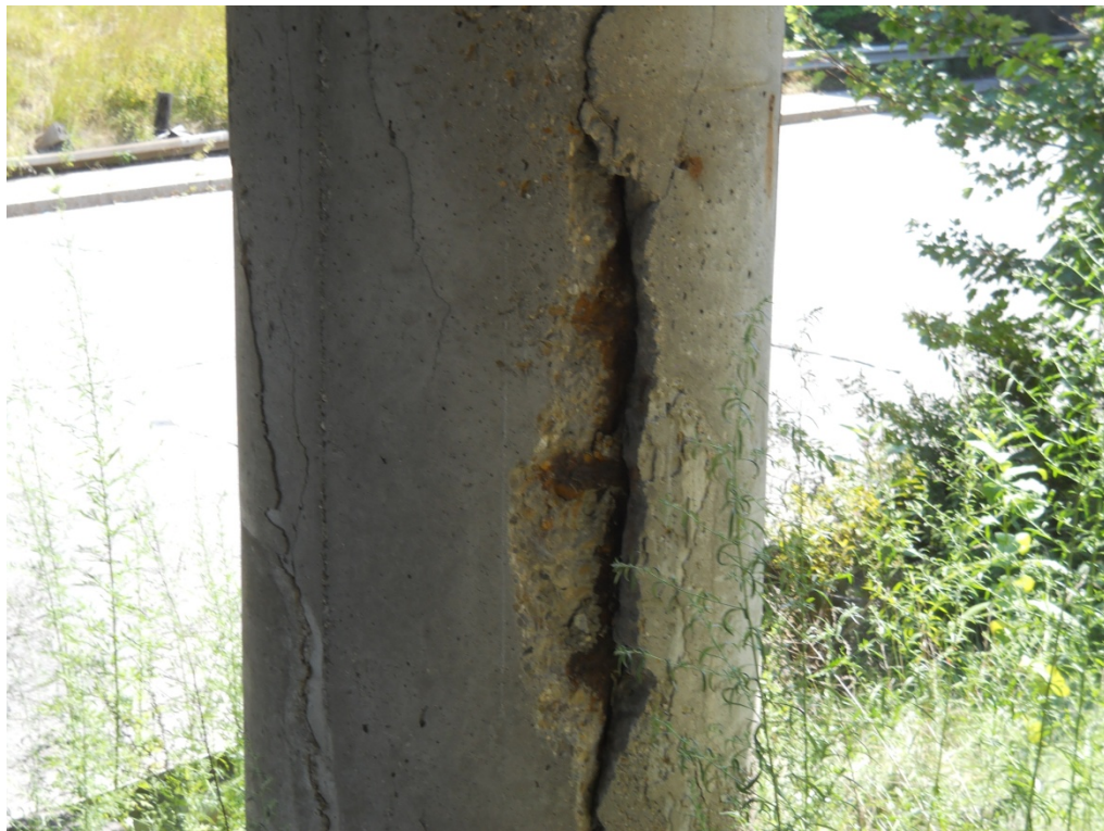
Figure 5: Severe spalling, cracking and separation of concrete cover on northern pier of NB Bridge.
