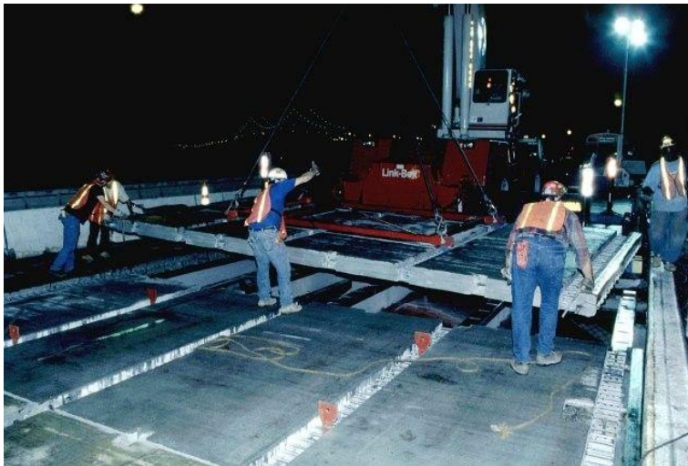
Figure 13: Prefabricated deck sections being placed over supports, image taken from FHWA website.
