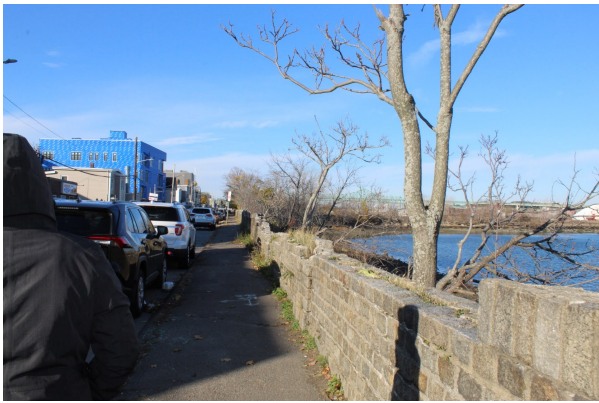
Figure 34. Erosion at Base of Wall
