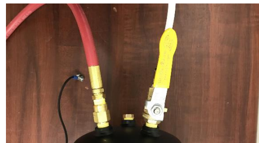
Figure 5B: Yellow valve handle parallel to air tank in open position
