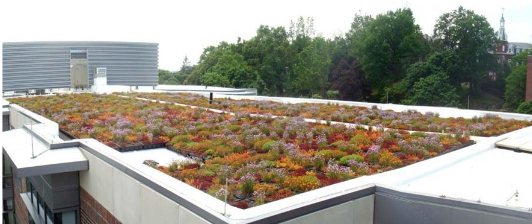
Figure 4.1: Nitsch/Maglioizzi Green Roof in Summer 2009 (Photo courtesy of Fred DiMauro, WPI, Assistance Vice President for Facilities)
