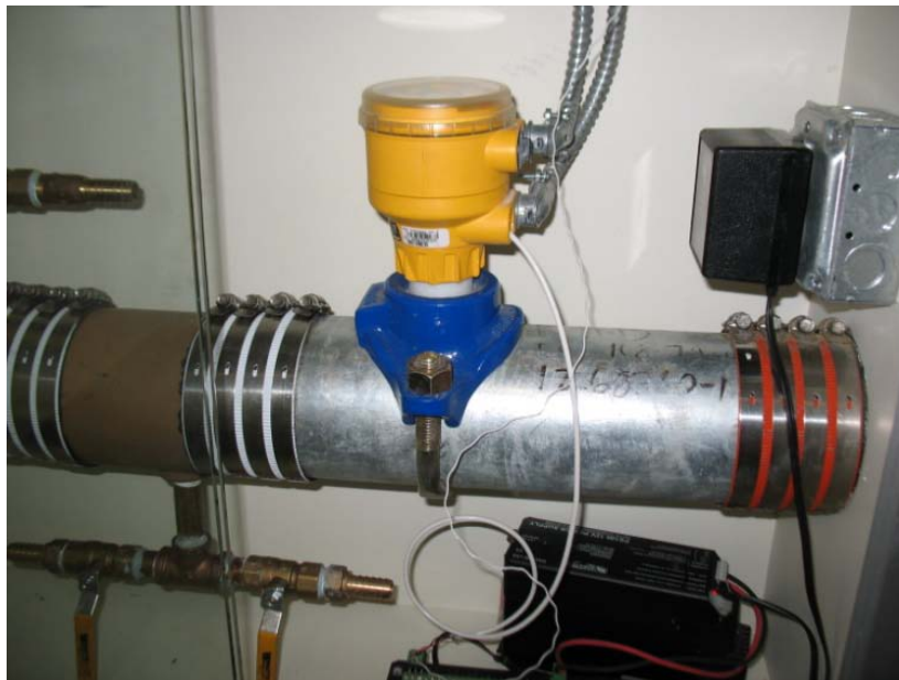
Figure 3.3: East Hall Green Roof Monitoring Station
