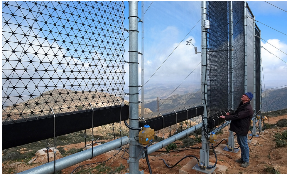
Figure 8: Fog-harvesting nets atop Mount Boutmezguida (Aqualonis, 2015)
