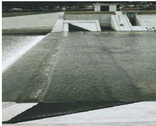
Figure 17 - Rubber dam deflated.
