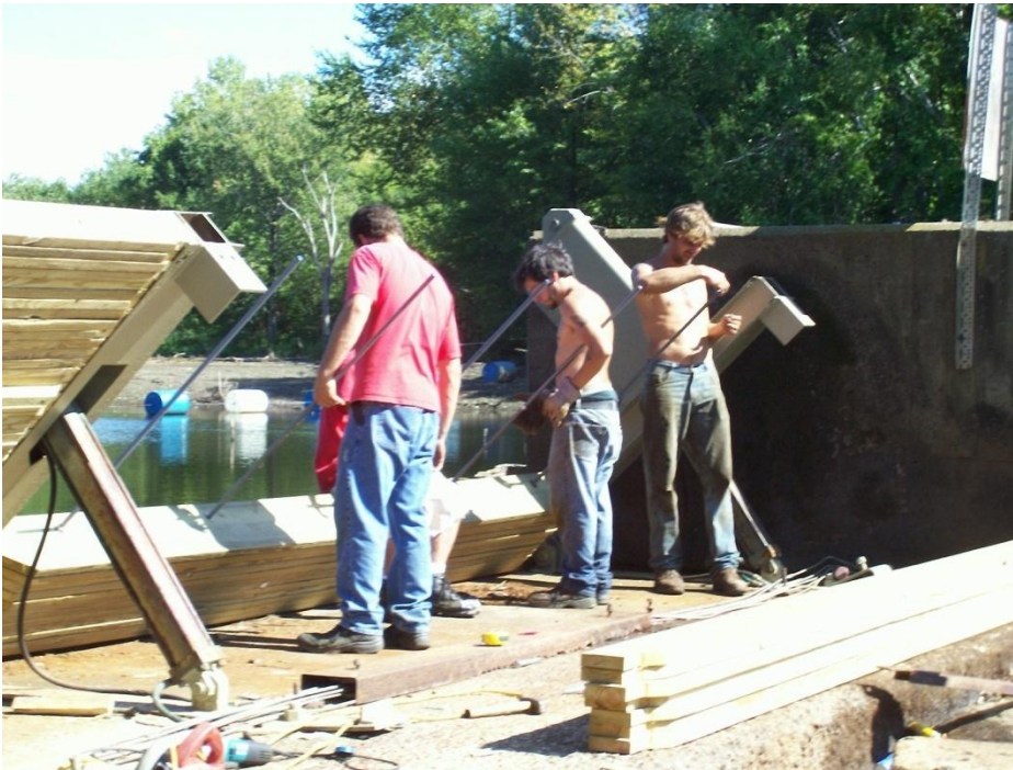
Figure Nine: Note the laminated panels being held together with stainless steel, threaded rod. This is a simple, durable method of construction
