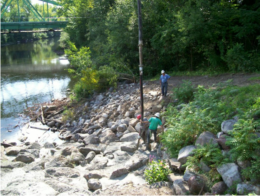
Figure Ten: The downstream riprap being stabilized with air entrained concrete. Up lift on the finished riprap was prevented with subsurface drains.
