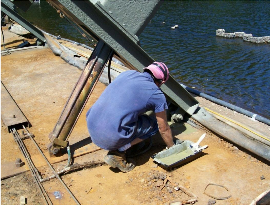
Figure Eight: A close up view of a hydraulically controlled, I-Beam, Needles.
