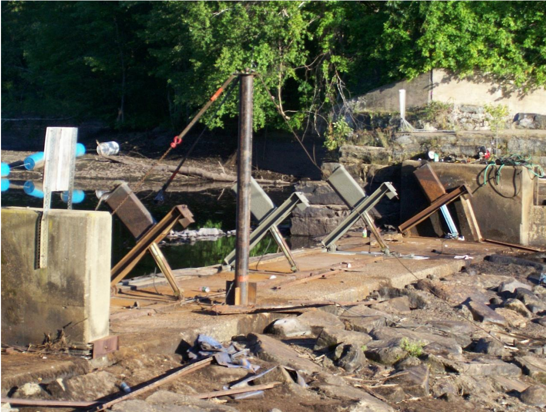
Figure Seven: Hydraulically controlled, I-Beam, Needles. Note the rectangular caps that the cylinders thrust on. The caps allow the boards to fully depress. They also protect the cylinder from debris flowing over the dam crest.
