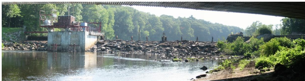
Figure Five: Summer of 2006 rehabilitation. Note all the wooden panels have been removed for replacement
