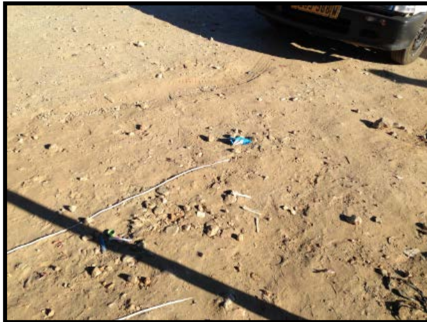
Figure 18: Buried electrical cables installed by local residents
