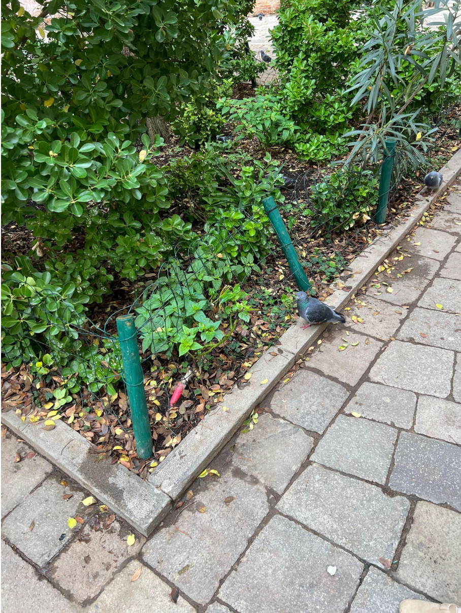
Green Space ID 278: Broken Fence.
