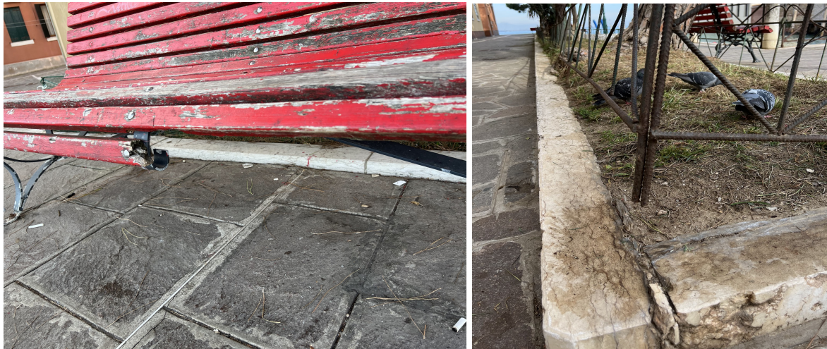
Figure 13. Example of a broken bench (left) and fence (right).
