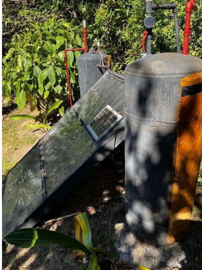
Figure 19. A solar water heater located on the ground.
