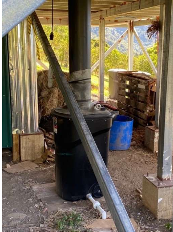
Figure 7. Composting toilet under a house, built on a slope.
