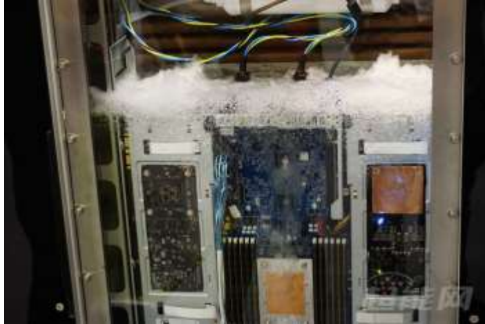
Figure 139: A photo of direct liquid immersion cooling [124]
