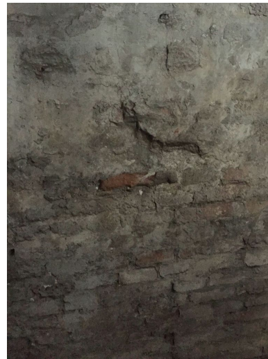
Figure 40.2: Crack in Sant'Alvise only a few centimeters
