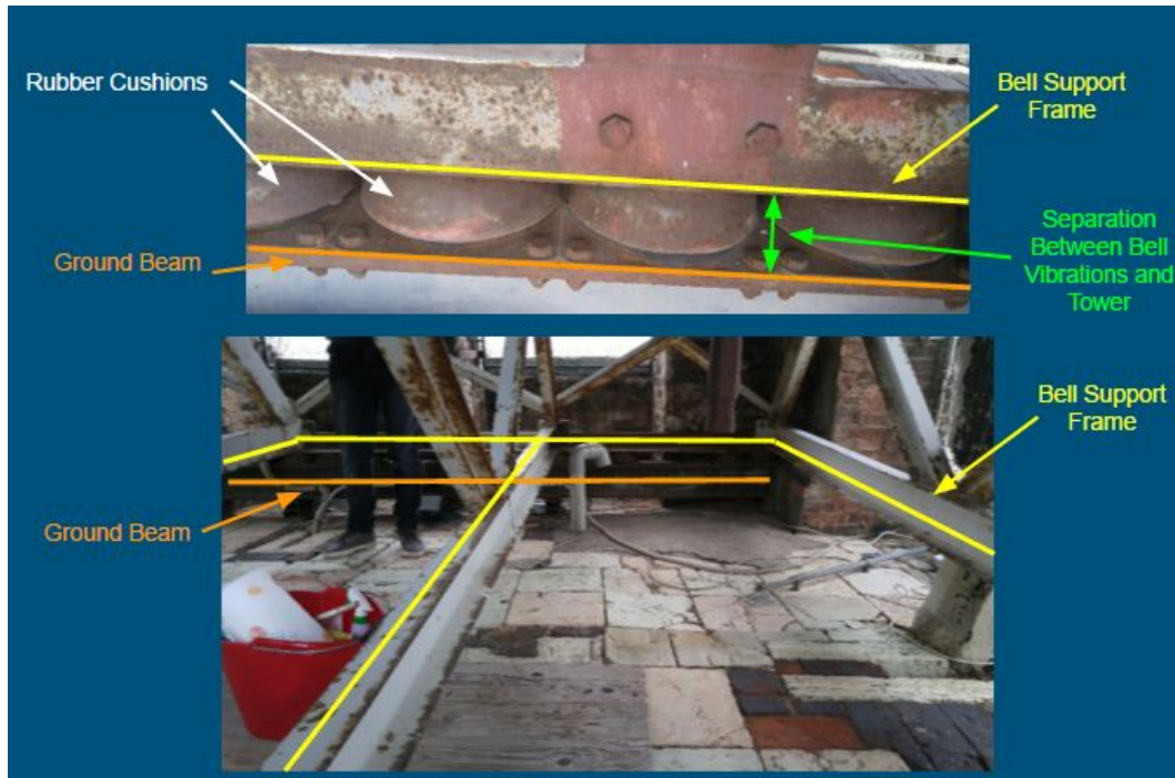
Figure 71: Vibration dampening device at S. Pietro
