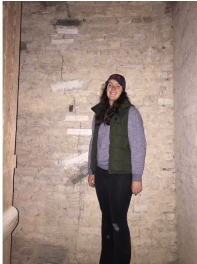
Figure 40.1: Crack in La Madonna Dell'Orto longer than a person
