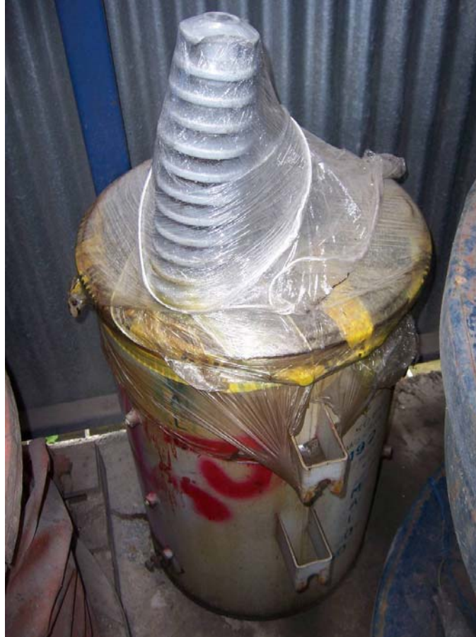
Figure 2: Image showing a transformer containing PCBs in ESPH's warehouse
