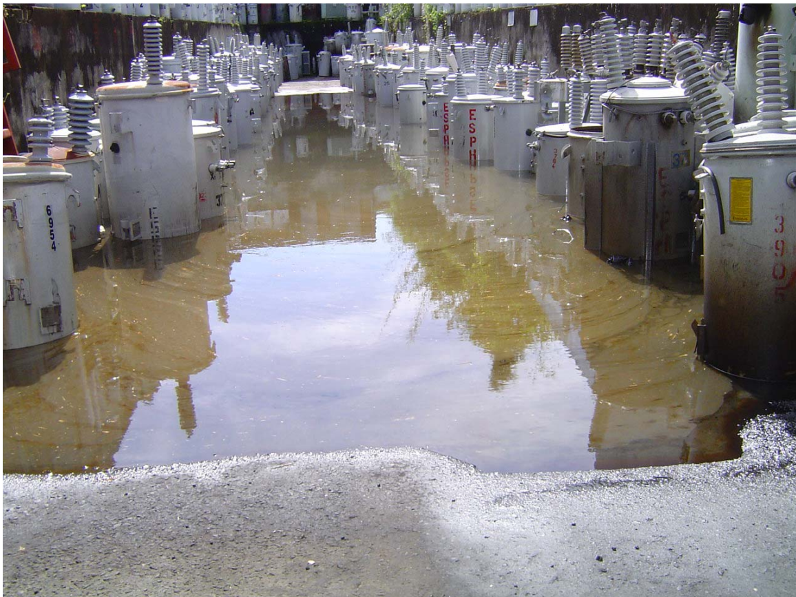
Figure 4: Image showing spilled transformer oil at ESPH's "The Patio" warehouse
