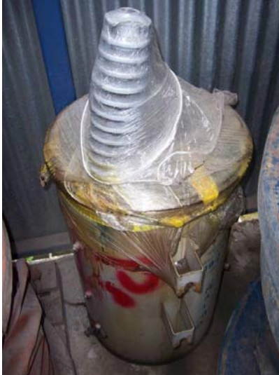
Figure 5: Image showing a transformer containing PCBs in ESPH's Warehouse B
