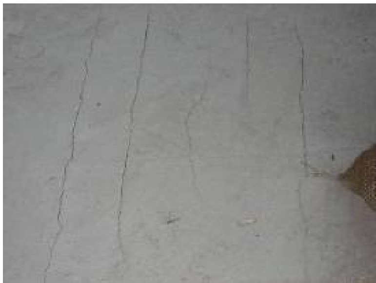
Picture 8: Second Floor Shrinkage
