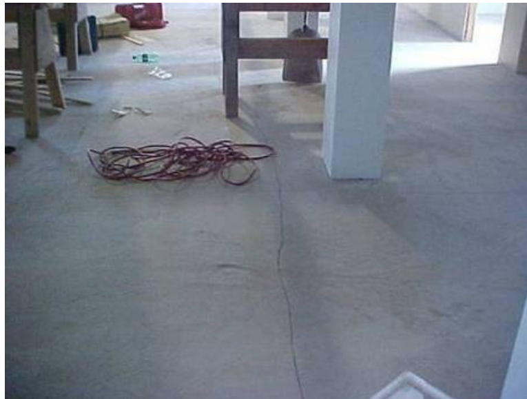
Picture 7: Tension Crack on Fourth Floor
