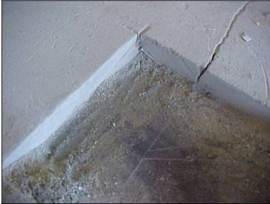
Picture 11: Tension Crack and Wood Floor
