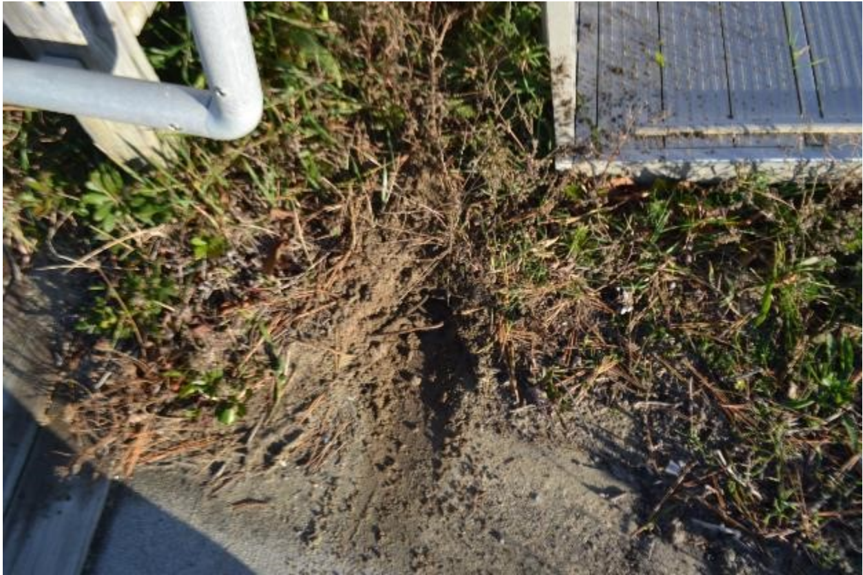
Figure 23: Overgrown Grass Around Bathroom at Dionis Beach
