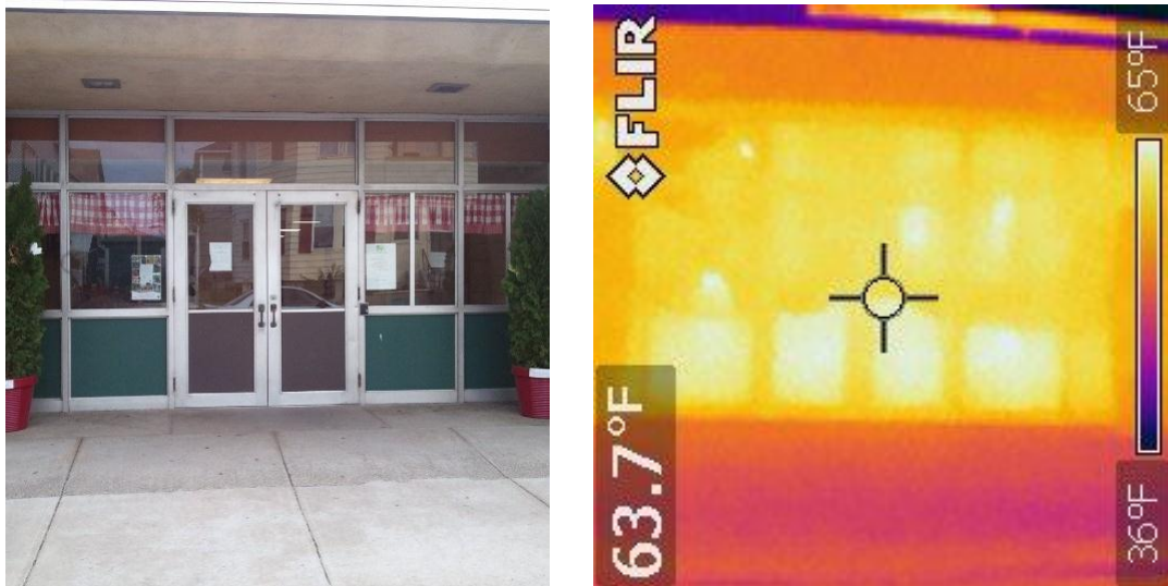
Figure 26. Main doors of the 1960 building (outside). Picture on left, thermal image on right.
