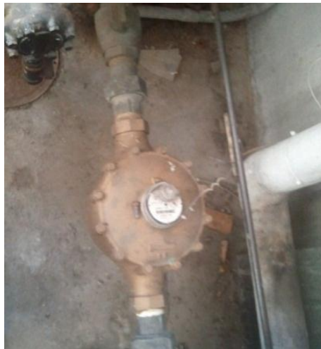
Figure 21. Water Meter located in 1960 building boiler room.
