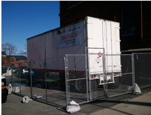
Figure 17. Temporary boiler in front of the 1890 building.
