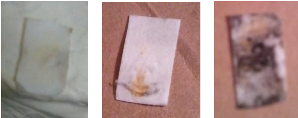
Figure 45. Lead Test Strips from 1890 building: on left, classroom wall paint; in middle, utility wall paint; and on right, pipe.
