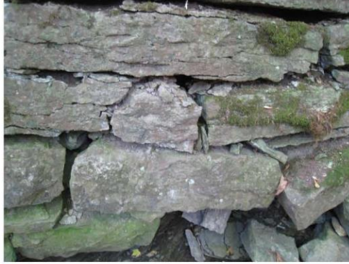
Figure 10: Existing abutment worn over time by cracks and erosion
