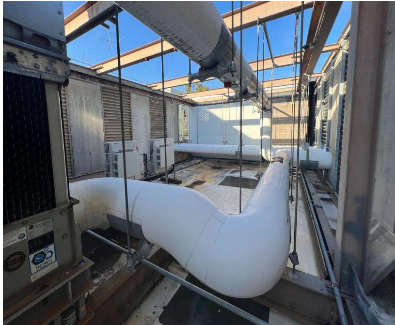
Figure 18: Interior of the mechanical penthouse screen wall showing unused space left over after the 2016 renovation.
