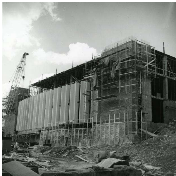
Figure 3: Construction photo of the Gordon Library showing the precast concrete fins being installed (Library Archives).
