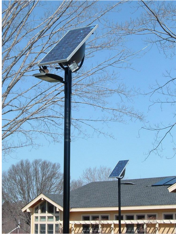
Figure 19: Stand-Alone PV Light at GRWECC
