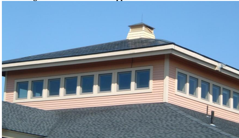
Figure 18: PV Panels on Uppermost Roof of GRWECC
