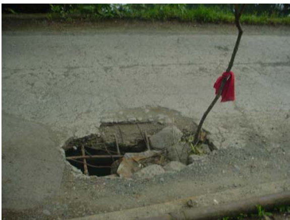
Figure 10: Dangerous road conditions
