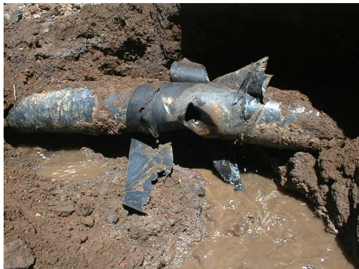
Figure 2: Oleoducto (oil pipeline) puncture
