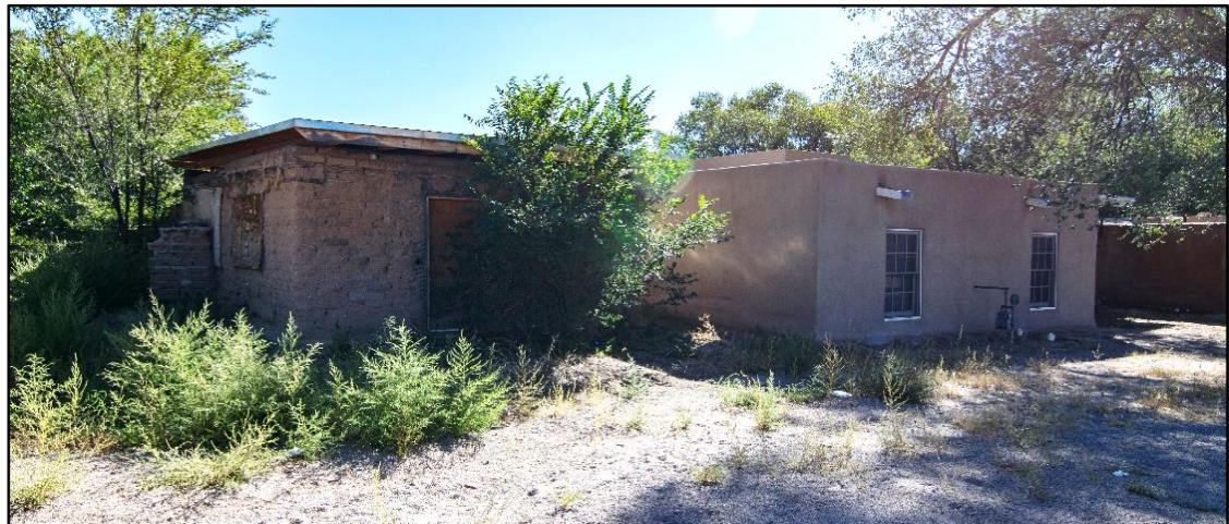
FIGURE 1: A TRADITIONAL ADOBE HOME IN DISREPAIR SITS NEXT TO A RECENTLY RENOVATED ADOBE HOME
