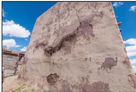
FIGURE 20: PHOTOGRAPH OF CRACK ON THE EXTERIOR OF OLD ZUNI MISSION
