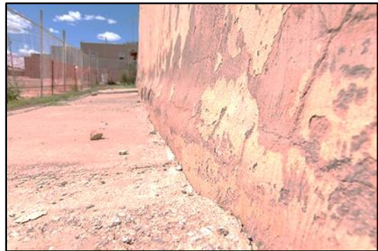
FIGURE 19: PHOTOGRAPH OF DAMAGE ON THE EXTERIOR OF OLD ZUNI MISSION
