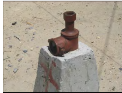
A Fire Hydrant in Mon-
