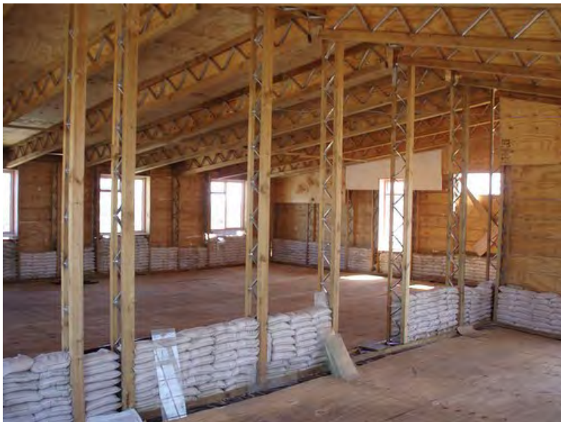
EcoBeams and sewn, filled sandbags utilized to construct the two-story Backpacker's Lodge in Monwabisi Park.
