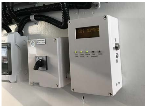
Figure 8: Control Panel at Entrance of MIH
